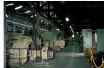
Interior of a Powerhouse
